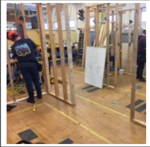
Lab environment with students achieving 2.5 meter separation.
