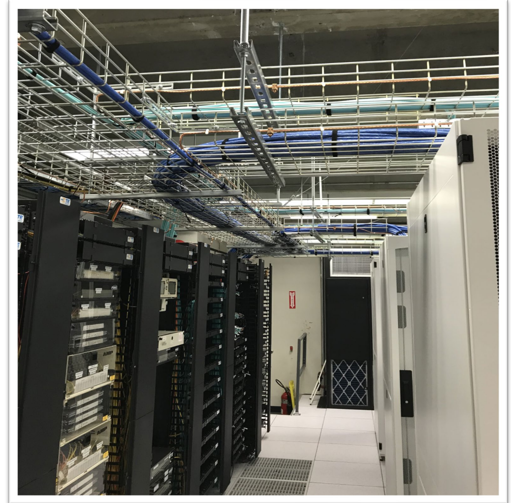
BCIT Central Data Centre (SE12)
